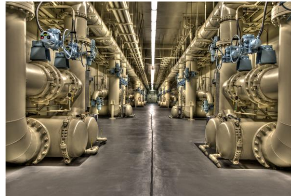
Treated at Quail Creek Water Treatment Plant
