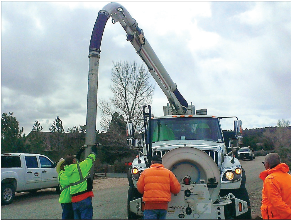
Crews operate vacuum trucks to remove nearly 17,000 gallons of sludge from Dammeron Valley's wastewater system in 2014.
